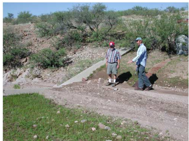
Figure 1. Illustration of the sediment accumulations upstream from a broad crested weir on watershed W-5 at Safford, Arizona. Sediment removal from the pond above the weir is required to maintain hydraulic flow conditions.
