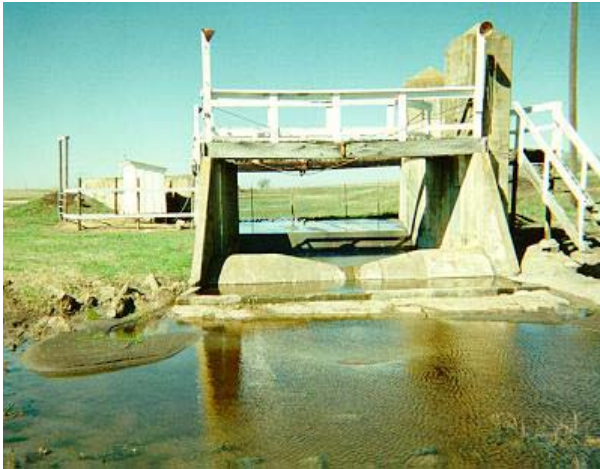
Figure 3. Flow control structure located on a 53.4 ha watershed.
