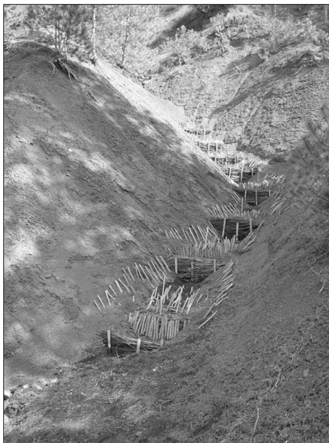
Photo 1. Optimal rehabilitation of an eroded gully with brush layers and brush mats on fascines (Photo by Freddy Rey)
